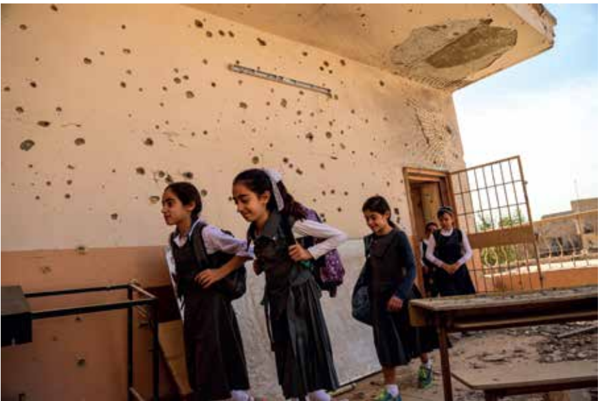
Damage from conflict is clearly visible at a school/ Ramadi, Anbar Governorate , Iraq/ Wathiq Khuzaie
