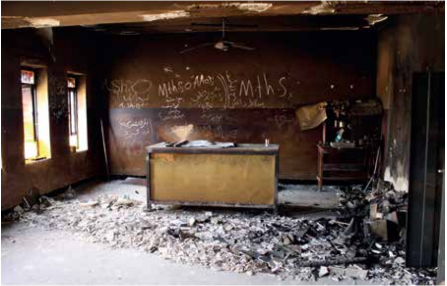
Destroyed school room at Gerver Secondary School/ the Zumar sub-district of Ninewa , Iraq/ Veronika Jemelikova
